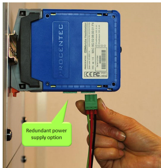
Powering the Head Station
